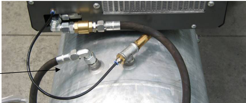
Illustration: control air hose at air receiver
